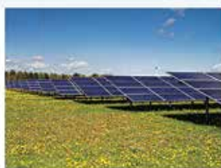
PV Solar Parks
