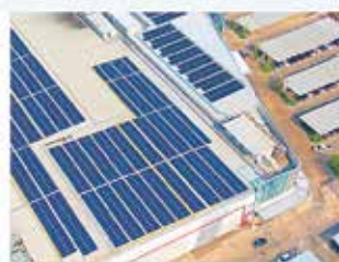
PV Solar Roofs
